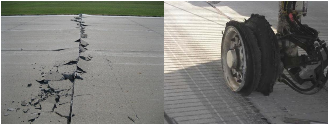
Figure 2-5. Pavement blowup and damaged aircraft in Ankeny Regional Airport runway (photo courtesy of Snyder & Associates, Inc./Polk County Aviation Authority).
