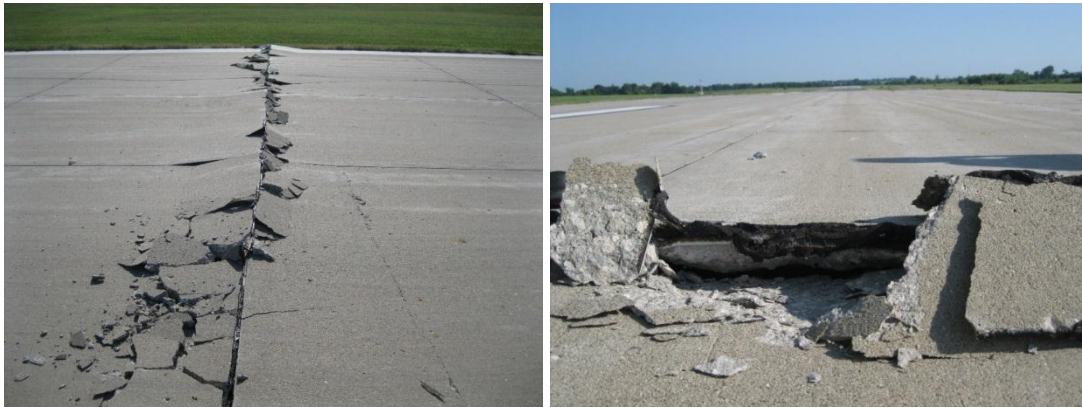
Figure 1. Blowup in Ankeny Regional Airport Runway (Photo courtesy of Snyder & Associates, Inc./Polk County Aviation Authority)
