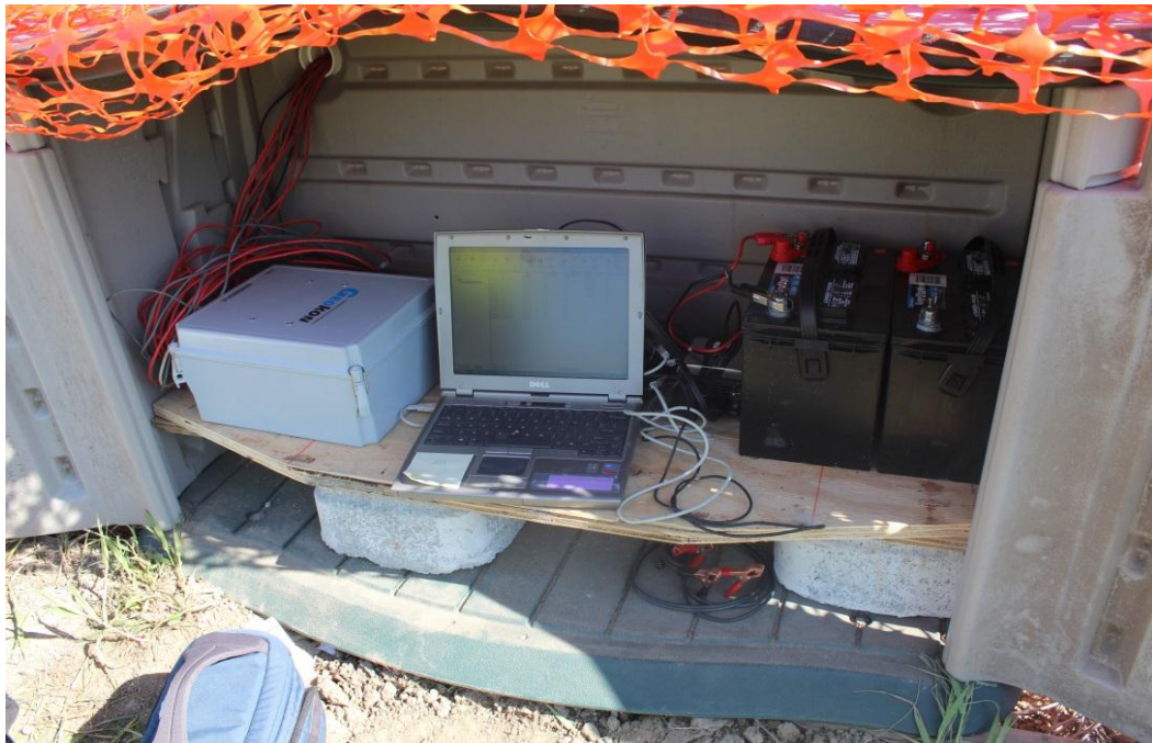
Figure 3-16. Data Acquisition System (DAS).
